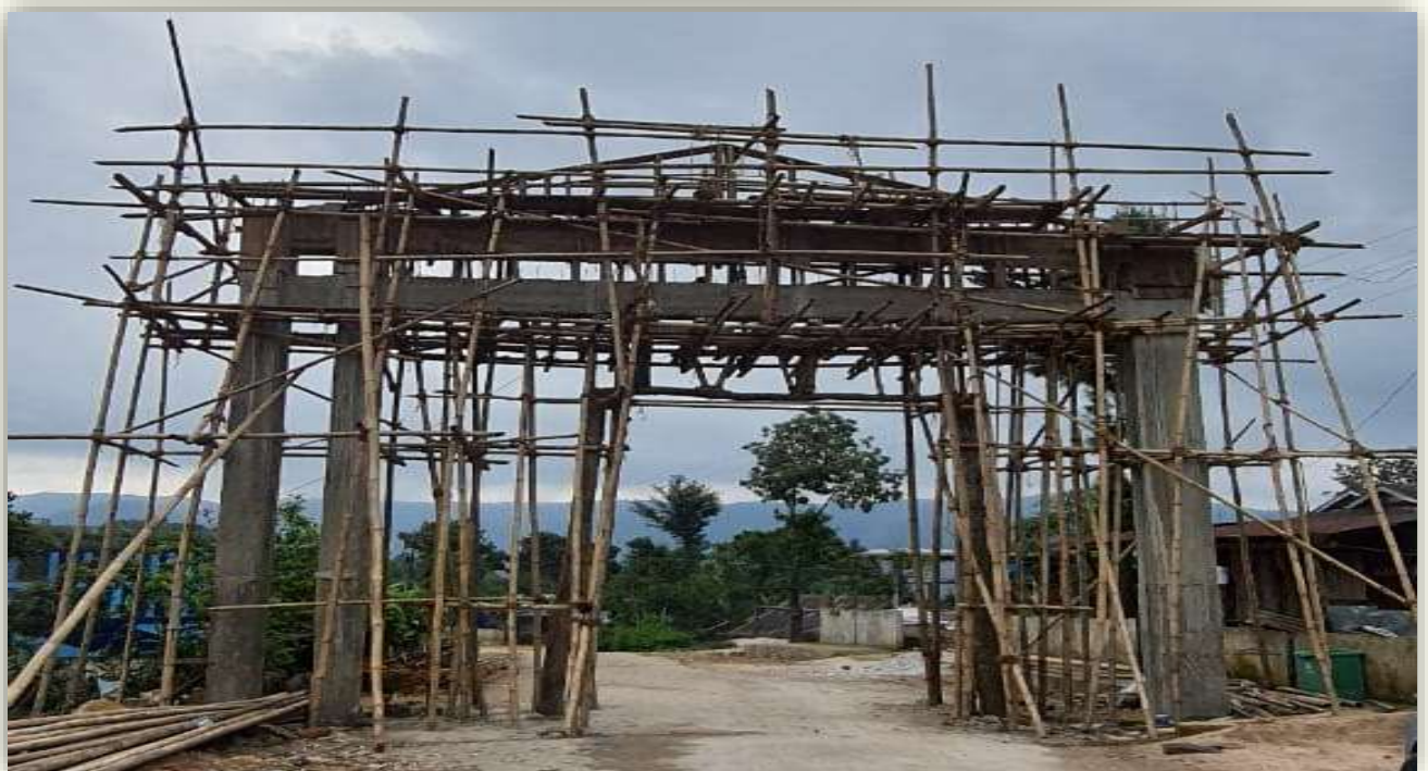
Final stage for the Construction of the Entrance gate for Kongthong village in association with AARIS LLC
